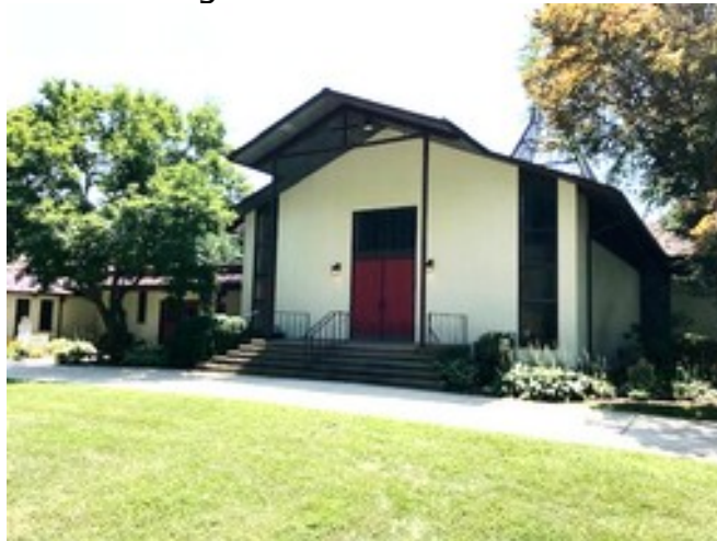
Picture of front doors that need replacing.
