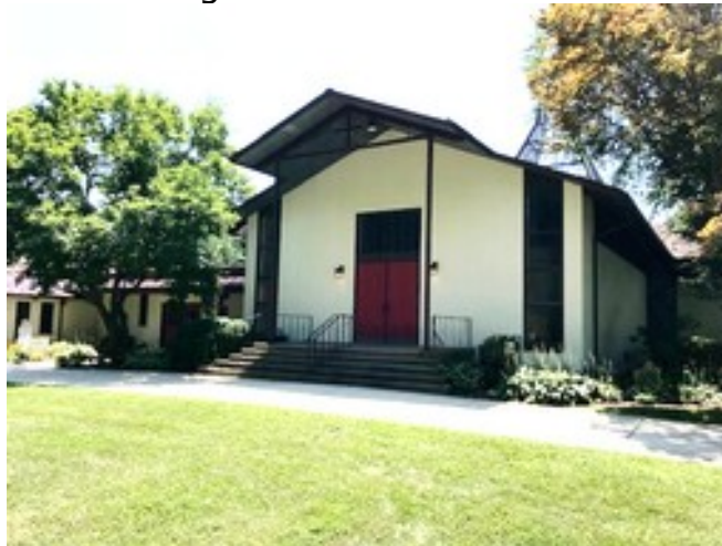
Picture of front doors that need replacing.
